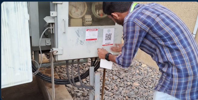
NFPA 70E labels, applied at site
